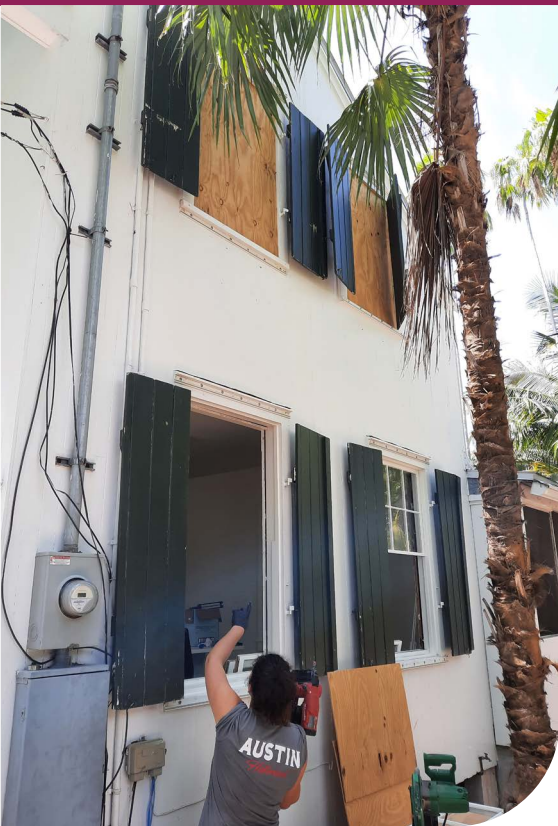
The team from Austin Historical is installing newly restored windows in the Elizabeth Bishop House in Key West.
