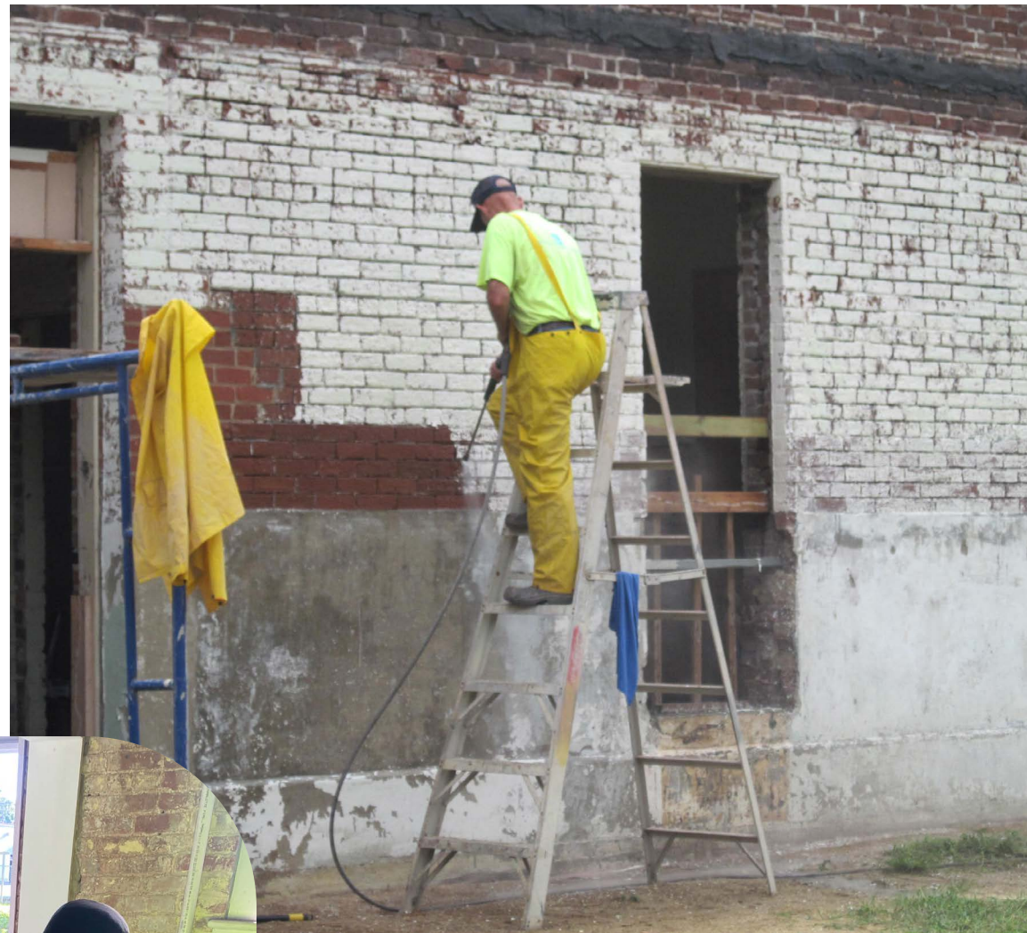
Removing paint from historic brick at the St. Augustine Waterworks. Credit: Jennifer Wolfe
