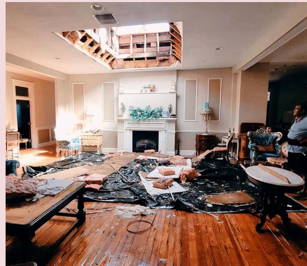
Water intrusion from Hurricane Ian caused structural damage in this home, resulting in the collapse of their ceiling. Credit: Florida Trust
